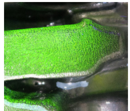
Figure 5: Thermally induced cracking Source: Kind & Co., Edelstahlwerk, GmbH & Co. KG
