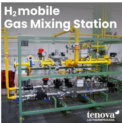
Picture 2: Tenova LOI Thermprocess mobile Gas Mixing Station
